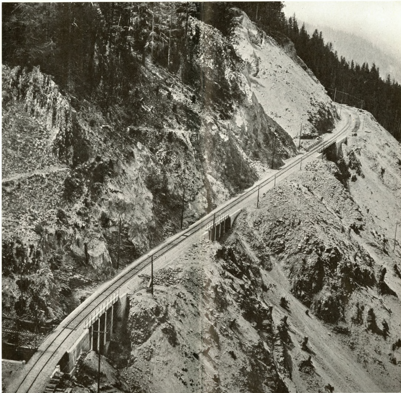
C ONCRETE slab bridges are used in the heavy construction work on the new Cascades Line. Railroad engineers cut through solid rock and hewed a great lane through forests in building the road. This view is on the west side of the Cascade range in Salt Creek Canyon near the summit.
