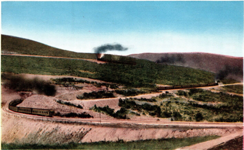
4393. Denver & Rio Grande Trains Ascending Soldiers Summit, Utah, over the New Double-track Line
