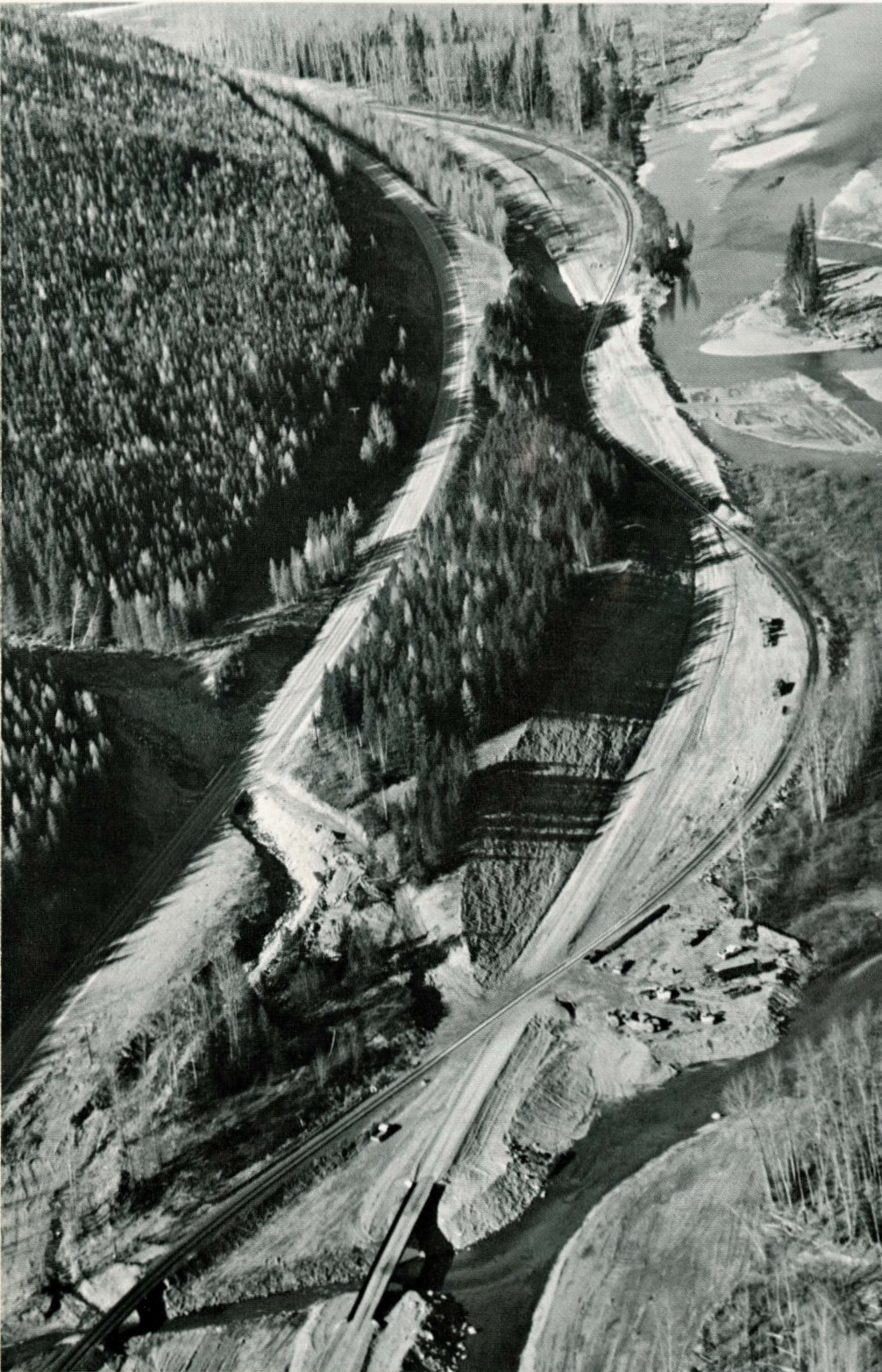
Two significant track improvements were made in the Montana Rockies in 1965, considerably reducing main line curvature in the Summit and Red Eagle areas. This aerial view of the Red Eagle project shows where three curves were eliminated in a distance of 8,575 feet. U. S. Highway 2 parallels the rails here.
