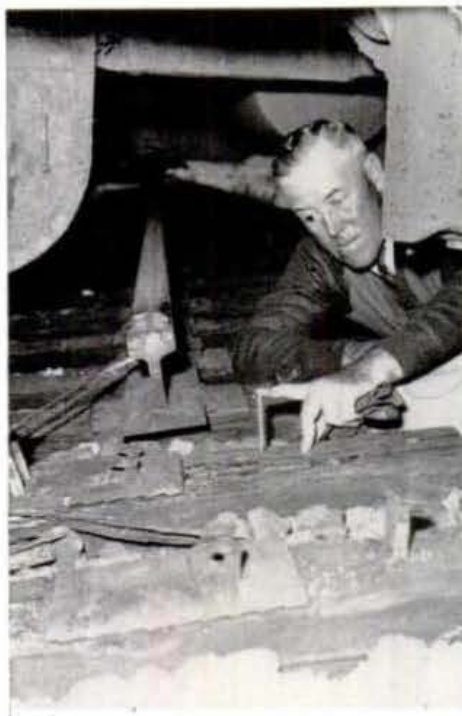
Sabotage was effected by moving rail out of line. Tie plate and signal cable at left show angle of displacement.
