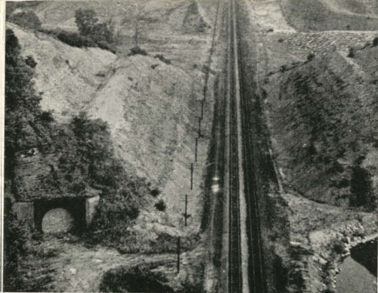
New main line, in cut through the hills near Cadiz, Ohio. The entrance to the old tunnel, with its restrictions on the size of freight car shipments, is in side of hill at left.
